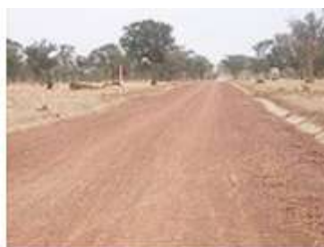
A road constructed by the Millennium Villages project to connect the cluster to the hospital and markets
