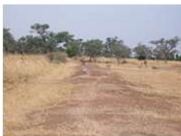
Road conditions in Mali before the project
